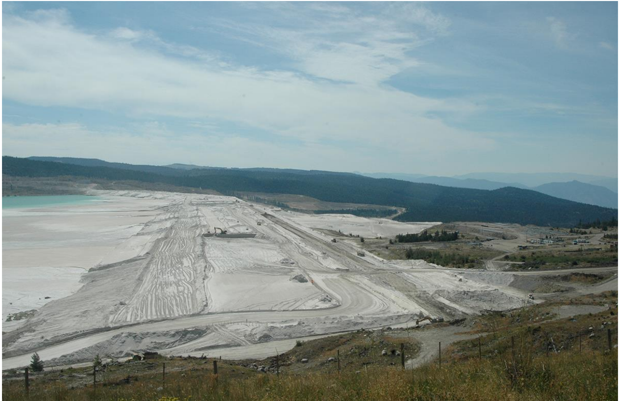
Copper-mine dump and landfill at „Highland Valley Copper“, Logan Lake, B.C. , Canada © chrisbuerki-photography.net , 2015
